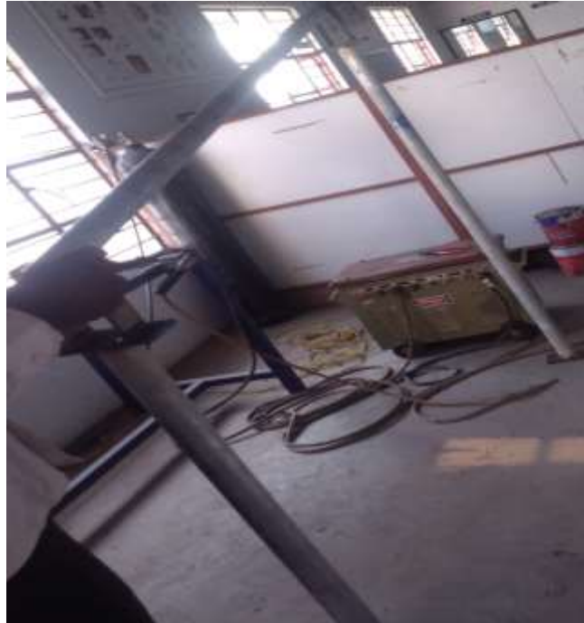
Fig.5: Supporting Stand for the Photovoltaic Panel
